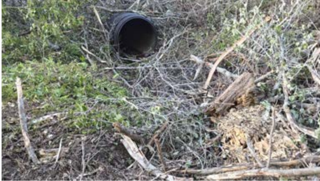
Image 5: Intense debris left before pipe culvert on Stream 3 north of Eskimo Hill Road. Photo taken May 31st.
