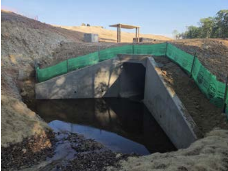
Image 13: Ponding on North side of the new access road, near S1-3. Photo taken June 21st.
