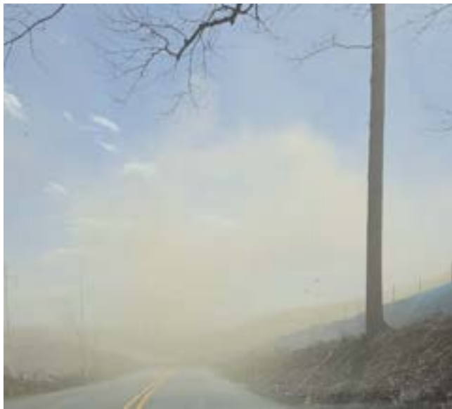
Image 12: Sediment blowing onto Eskimo Hill Road from STC construction area pictured on the right. Photo taken March 23rd.
